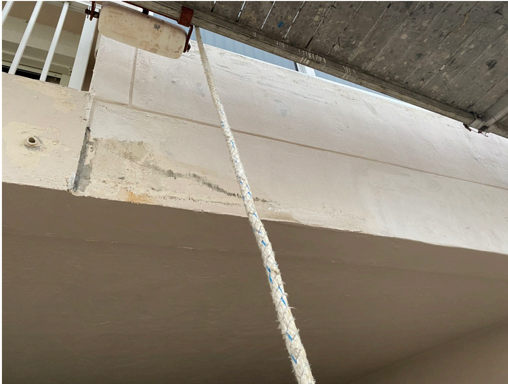
Picture 4: Crack in wall below Unit 108
